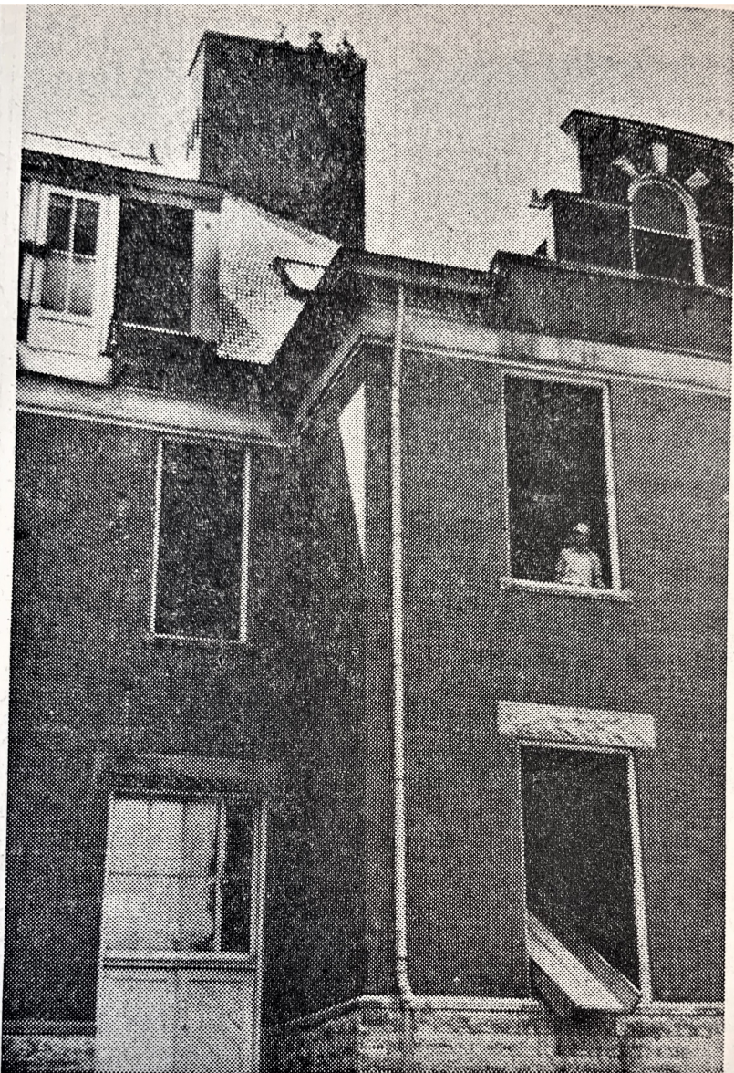
CHIMNEY SWEEPS —Work of removing the huge brick chimneys atop the old Washington School has been started by the Cupp Construction Company. Three men employed by the firm appear like three ants at the top of this chimney, located at the north end of the building. Another chimney at the south end will also be removed. Bricks from the chimney "ride" down a chute to the ground. End of the chute can be seen in the window at the right. (Staff Photo)
